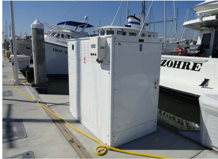
AMP Marina Sub Installed - Port of Bellingham, WA
