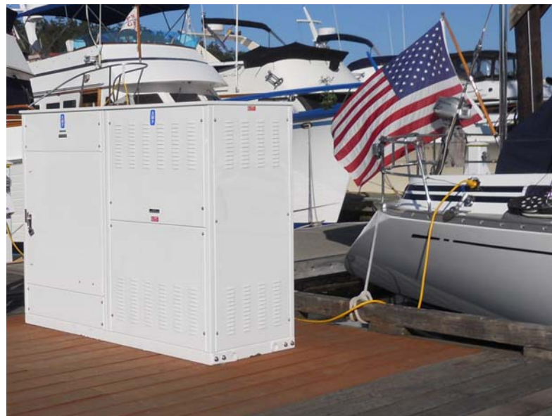
Substation w/ Side-by-Side configuration
